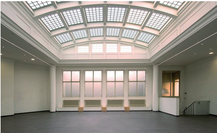
Galerie La Forest Divonne Bruxelles An exceptional Art Deco glass roof in the creative and trendy Saint-Gilles neighbourhood
